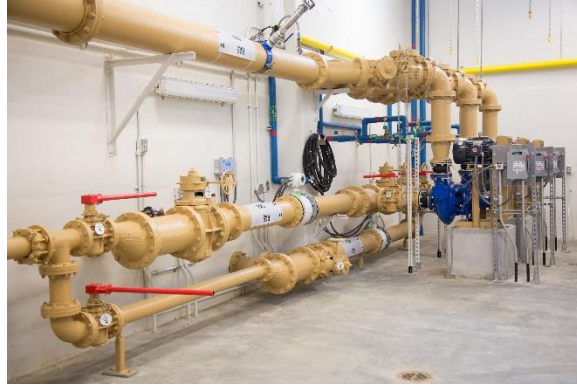
RAS Pumps and Piping
