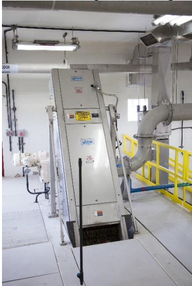
Influent Stair Screen
