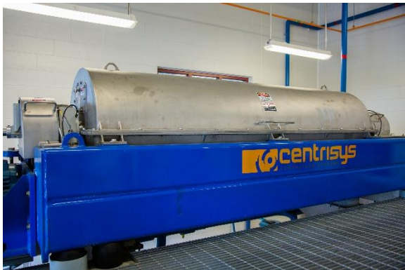
Biosolids Dewatering Centrifuge
