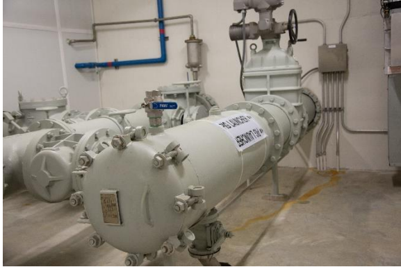
Pump Piping with Pig Launcher
