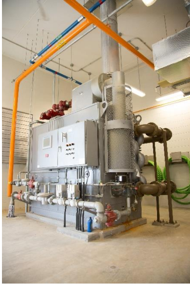
Combination Boiler/Heat Exchanger
